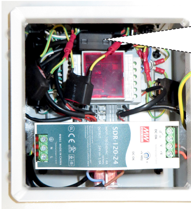
Control box interior
