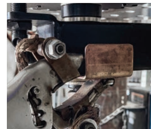
Built-in grounding point
